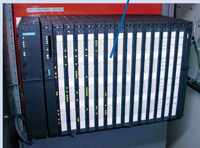
PLC 400 with Siemens S7 control system
