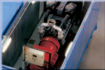
The diesel-generator set in the crane itself
