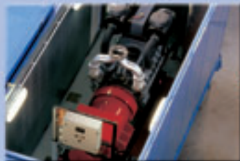
The diesel-generator set in the crane itself
