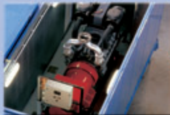
The diesel-generator set in the crane itself
